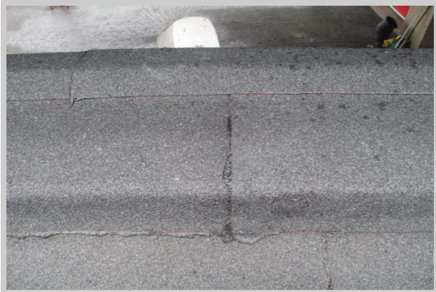
Perimeter and upstand details are well sealed, with a 5mm bead of bitumen extruding out of the laps.
