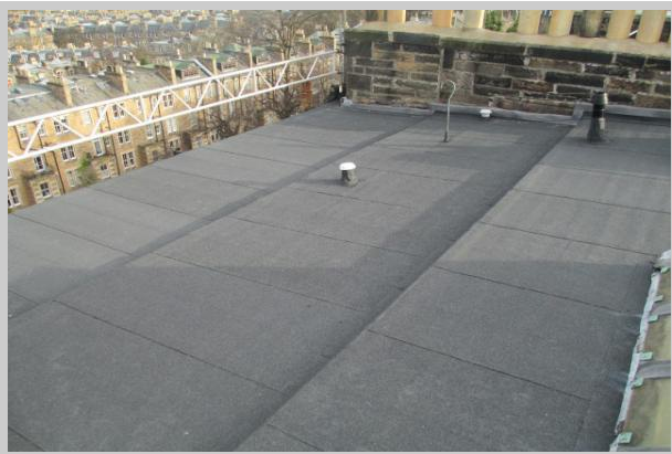
Overview of rear elevation. All works are completed to a high standard with all laps sealed.
