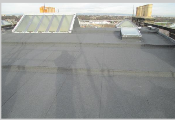
Neat felting work with a bead of bitumen extruding out all joints.
